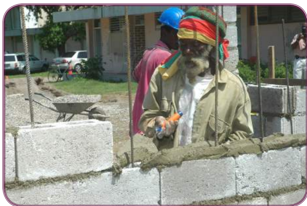
Community resident working on the Maxfield Park Professional Development Institute Day Care Centre.
