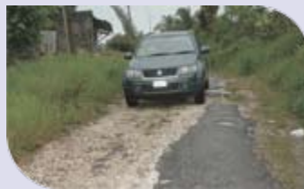
The existing Accompong road that is to be rehabilitated through funding from the Government of Jamaica.
