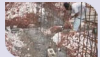
A labourer prepares the site for the relocation of the Montpelier Basic School
